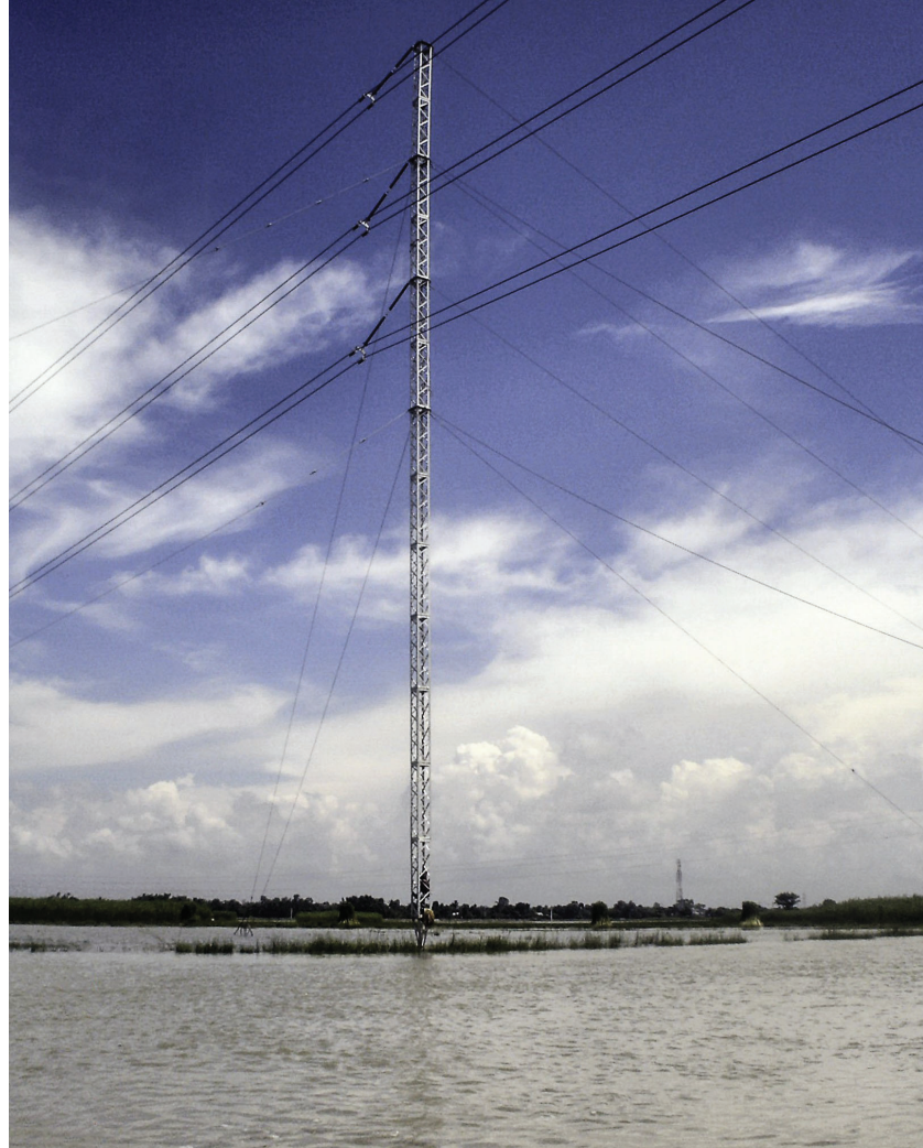
Figure 1. ERS Structure after flooding of the Patna River
