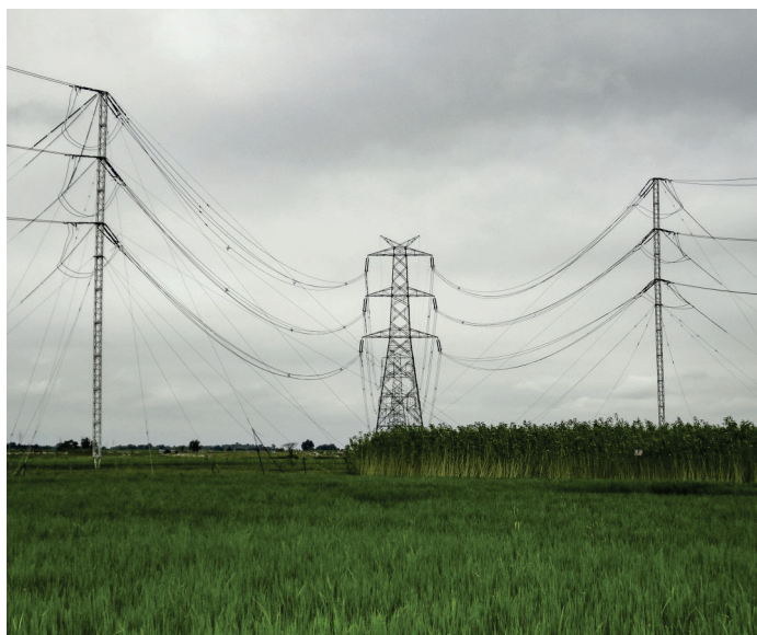
Figure 5. Two tension ERS structures pick up the two 400kV circuits from Tower 370 (looking west toward Purnea)
