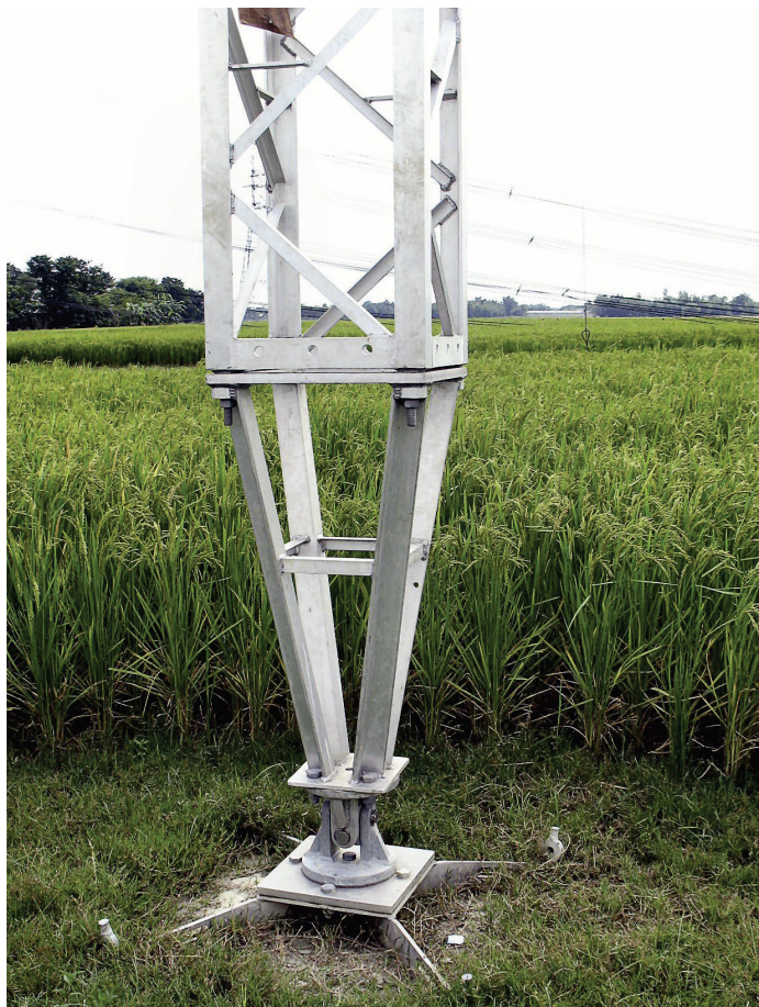
Figure 4. After flood waters receded, examination of the ERS foundations showed them intact.
