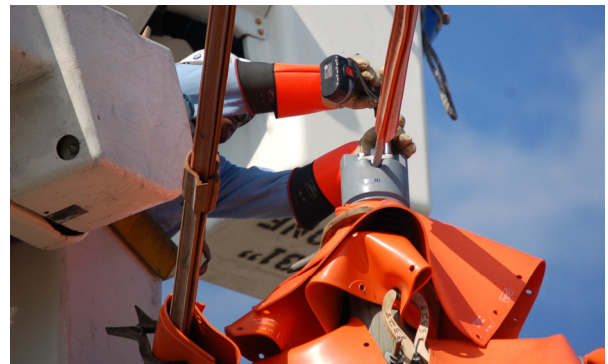
Figure 3. Example use of insulating blankets to shield sensor connector area from live line
