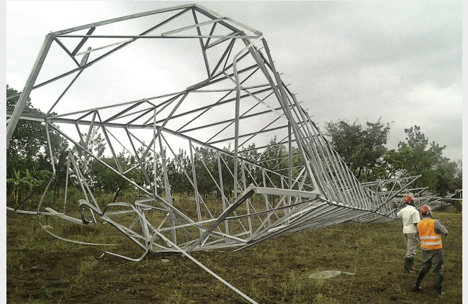
Collapse of a 132kV tower after bolts and crossmembers were removed to sell as scrap.
