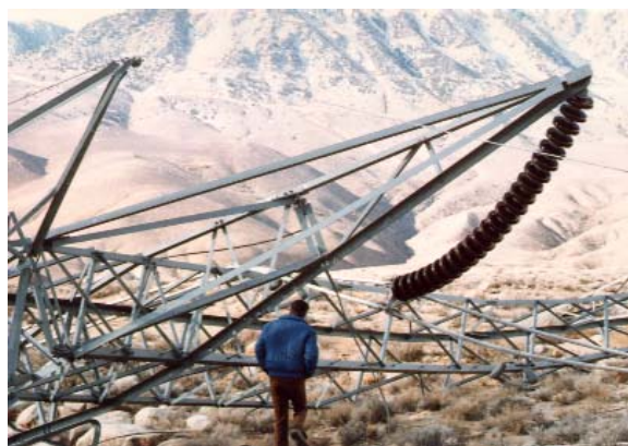
Figure 1: One of 16 cascaded 500kV DC Towers collapsed at the Los Angeles Department of Water and Power (LADWP) in 1988 due to High Winds
