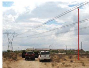
Figure 2: Location of LiDAR measurement taken from installed conductor monitor
