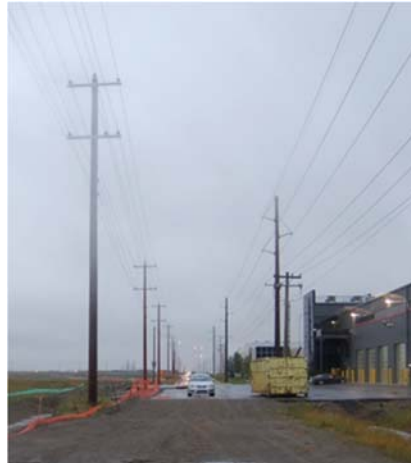
Figure 7: Commercial / Industrial environment conductor clearance monitor installation
