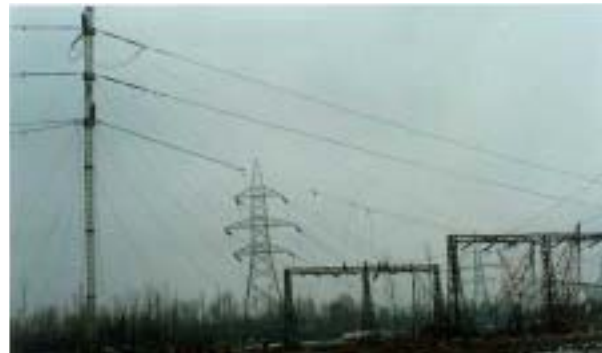
Figure 9 Two views of the almost completed 400kV ERS tension tower showing the span over the double circuit 220kV line.
