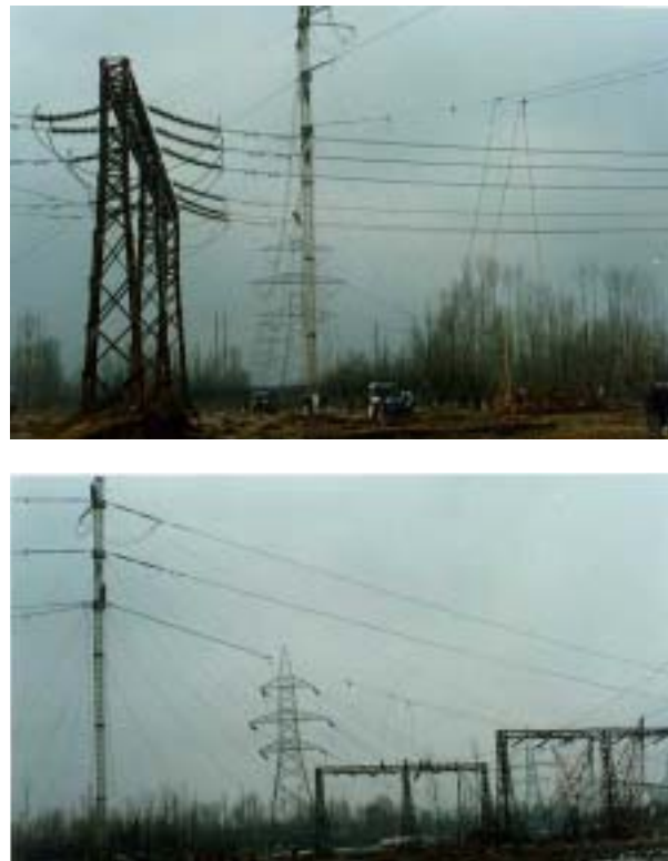
Figure 9 Two views of the almost completed 400kV ERS tension tower showing the span over the double circuit 220kV line.
