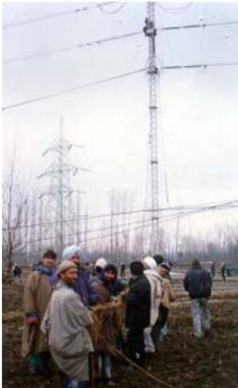
Figure 8 Erection of the 400kV single circuit 15-degree tension ERS tower using manpower to pull the two conductors of the bottom phase.
