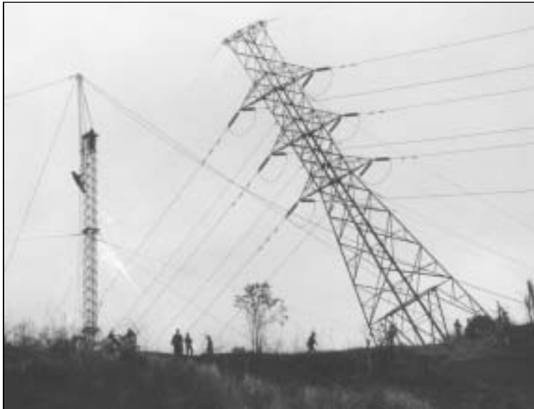
Figure 8 Vandals cut the legs of tension tower No. 44. This tower is located on the top of a narrow ridge. In order to keep the line energized, the conductor from one circuit was transferred to the ERS horizontal-vee structures while the other circuit was energized.
