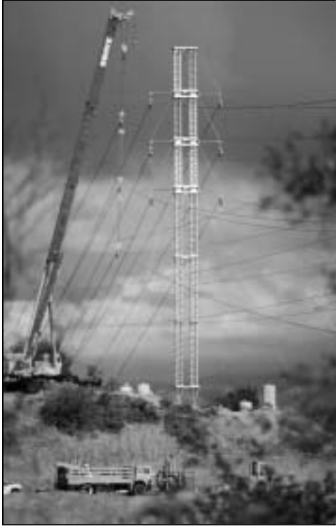
Figure 3 One 230kV circuit at the left is supported by the crane; two other circuits are supported by an IEEE Standard 1070 ERS. This double circuit 230kV ERS structure was designed for a narrow right-of-way.
